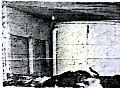
Storage and tempering tank which supplies the drinking cups in the Borglum barn. Part of water comes from rainwater piped from main barn roof.
